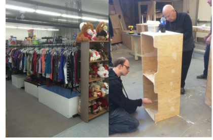
Students get to work! Construction class builds new storage boxes to replace the old ones.
